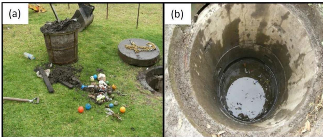
Figure 2-1: Example of asset failure attributed to ineffective maintenance: unreparable wet sump stormwater gross pollutant trap left un-maintained following construction 12 years earlier – (a) basket (b) sub-surface superstructure and wet sump (Author 2012).
