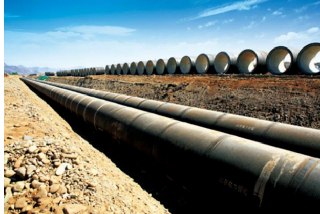
Figure 4.6 Water pipes of the SNWT in Beijing
