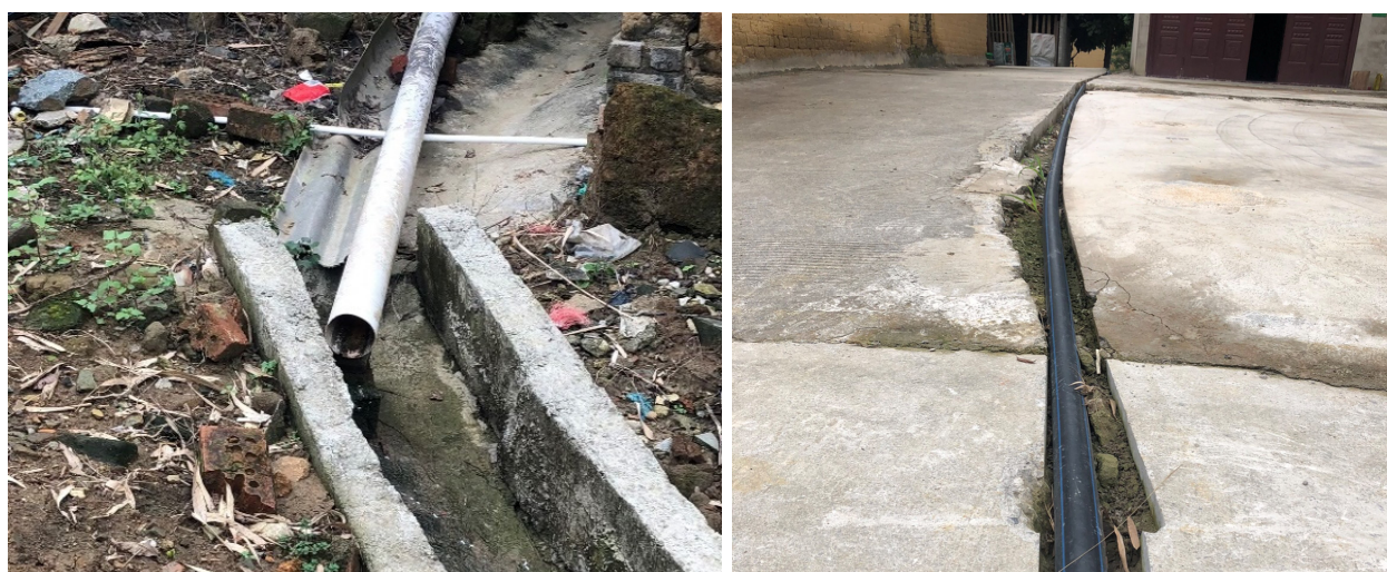
Figure 4. Sewage treatment facilities in Yanchi County. (Note: Photos taken by the first author.)
