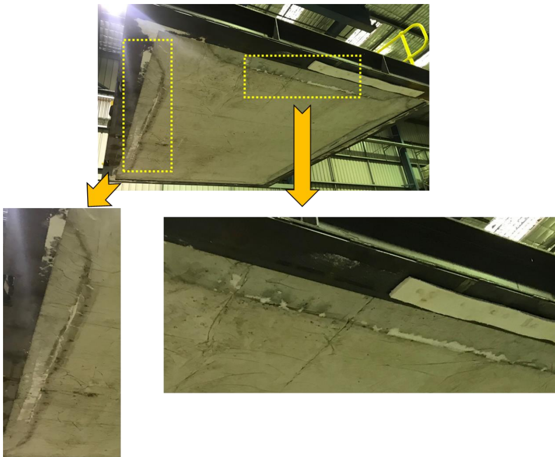
Figure 3.15: The exposed surface of the specimen after the test
