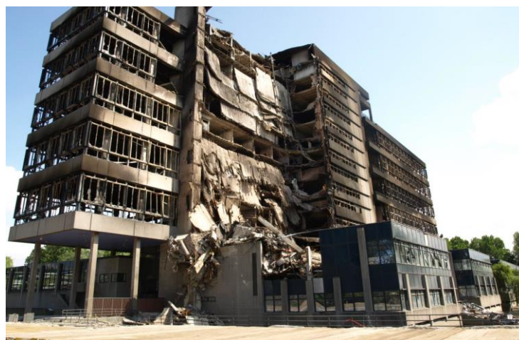
Figure 1.4: Partial collapse of the Architecture faculty building at Delft University of technology in 2008 (Kirk, 2010)
