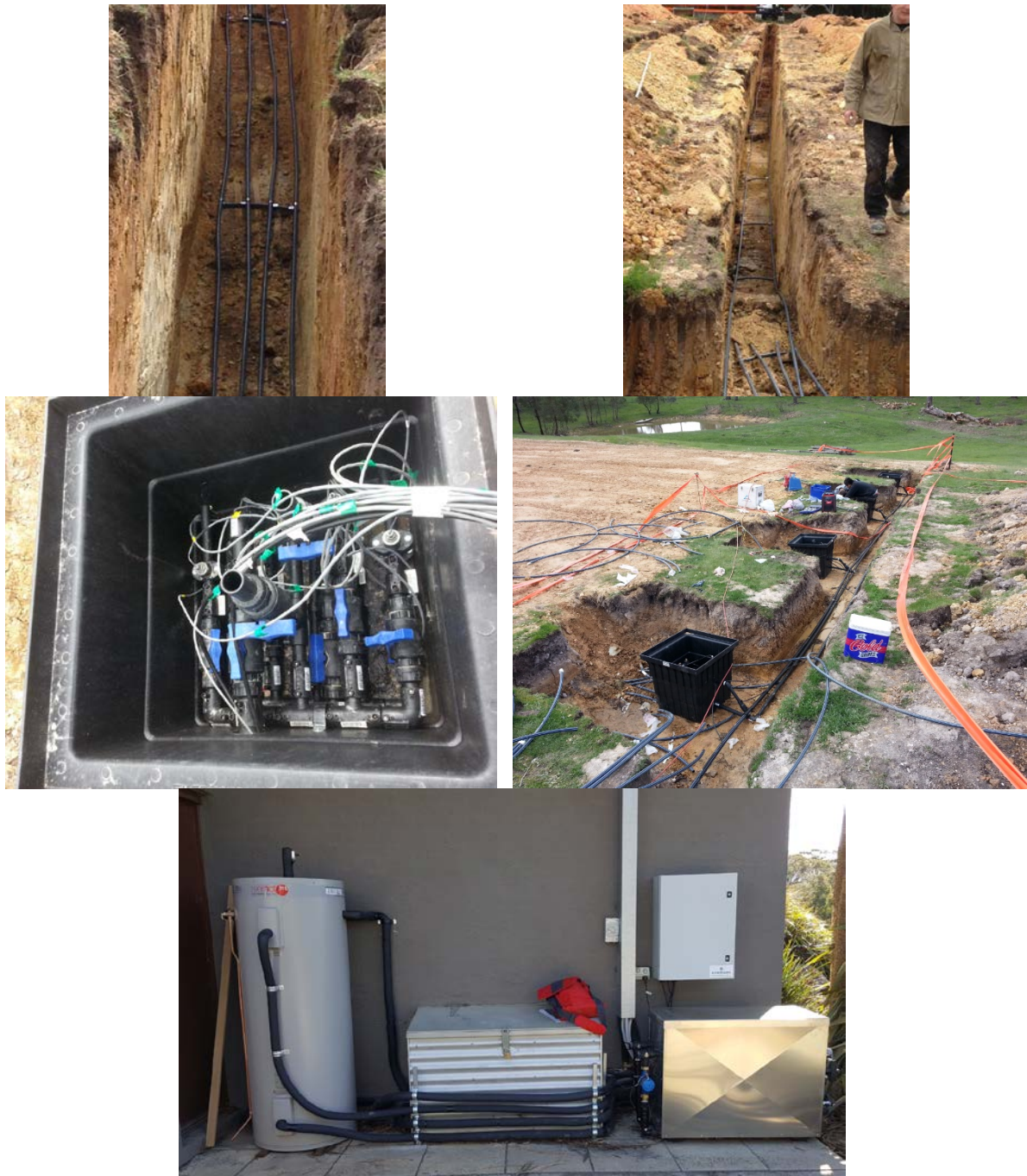
Figure B-5: (top row) installation of ground heat exchangers, (middle row) installation of thermal response test pit and instrumentation, and (bottom row) set up of heat pumps and data logger
