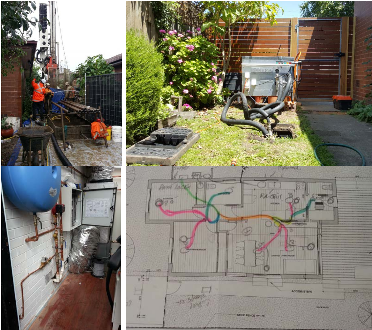
Figure B-26: (top row) installation of ground heat exchangers and thermal response test conducted in one of the boreholes, (middle row) heat pumps in the plant room and schematic of ducting installed
