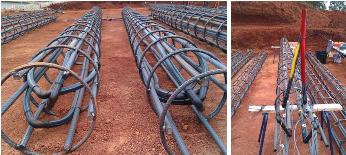
Figure B-42: (left) energy piles to be installed and (right) with instrumentation
