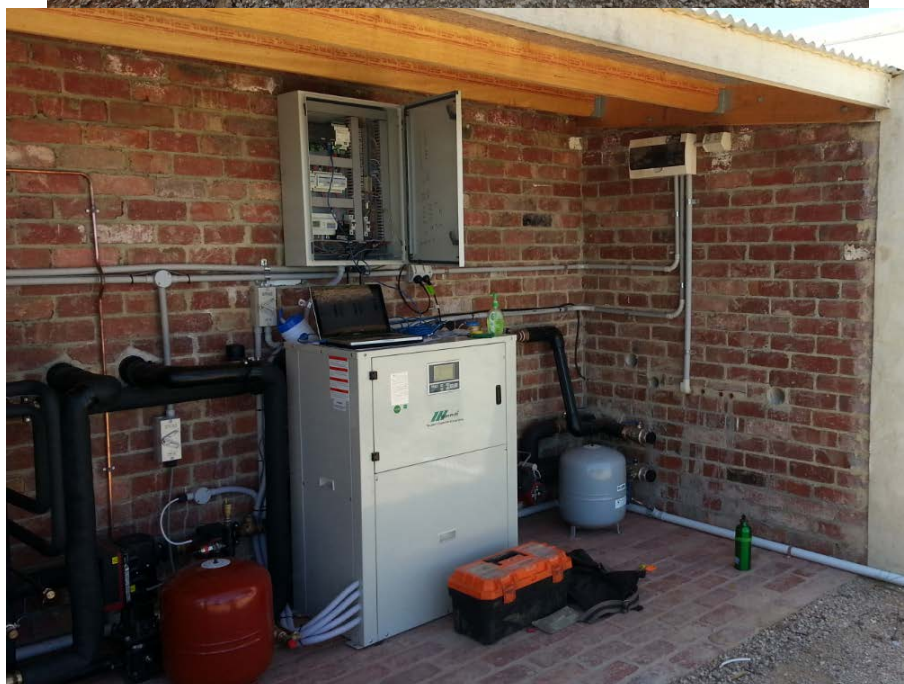
Figure B-34: (top row) trench where the ground loops were installed, and (bottom row) heat pump and data logger set up
