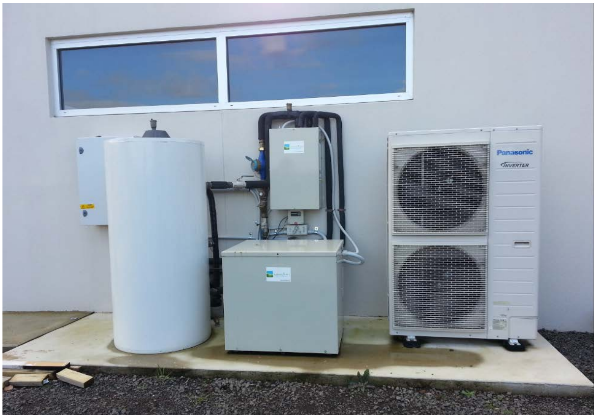
Figure B-33: Heat pump and water tank installed
