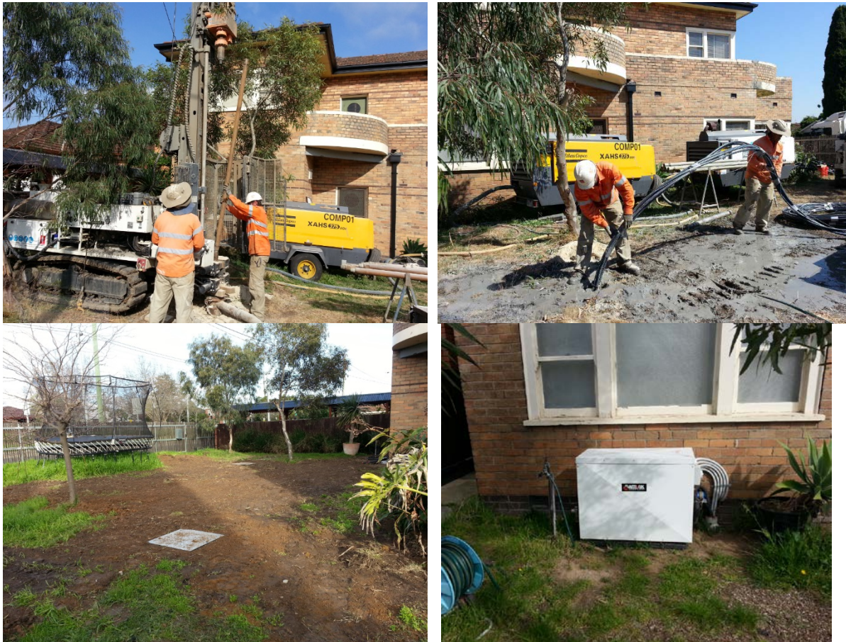
Figure B-51: (top row) drilling and installation of ground heat exchangers and (bottom row) location of thermal response test pit and the heat pump
