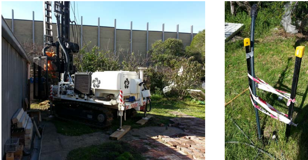
Figure B-46: (left) drilling of ground heat exchangers and (right) ground heat exchangers installed
