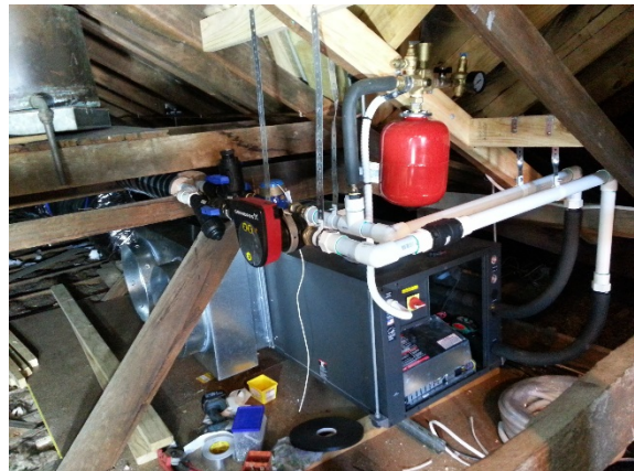
GSHP and circulation pumps in the roof attic at Cheltenham 1
