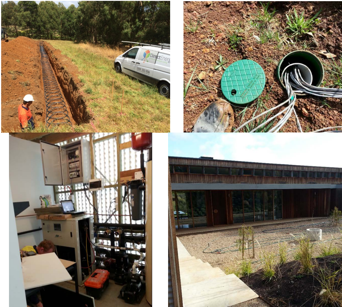
Figure B-37: (top row) slinkies ground heat exchangers installation and instrumentation (bottom row) heat pump and data logger set up and the property that is heated and cooled
