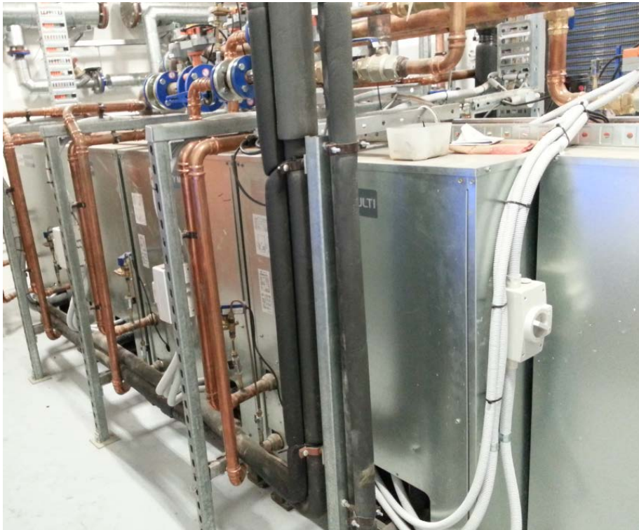
Figure B-9: Heat pumps installed inside the plant room
