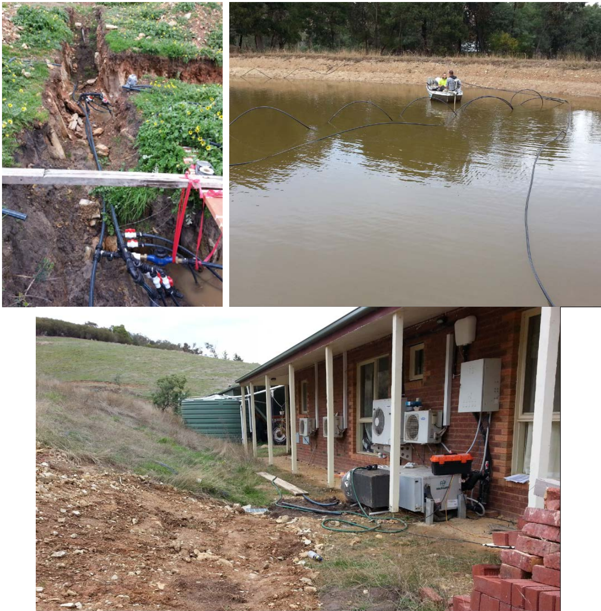
Figure B-48: (top row) header pipes for horizontal ground heat exchangers and installation of pond loops, and (bottom row) heat pump and monitoring equipment
