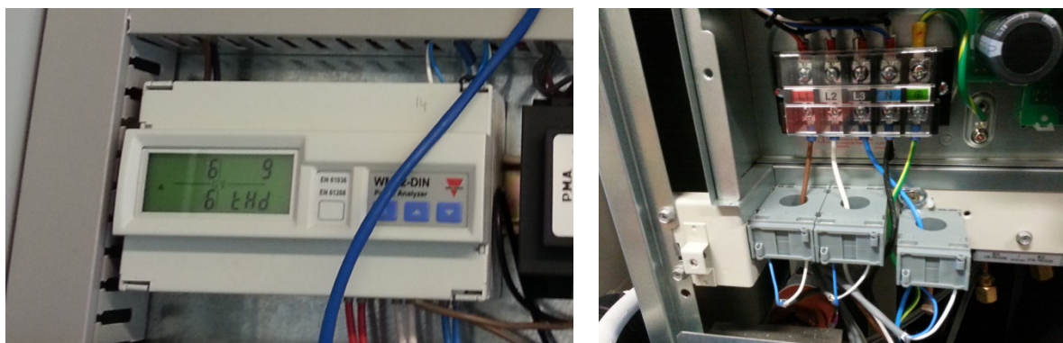
Figure 3-7: Energy analyser and current transformers used to measure the power consumption of the GSHP system: a) for a single phase system, b) for a three phase system
