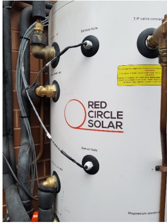
Figure B.21: Temperature measurement of the thermal storage tank
