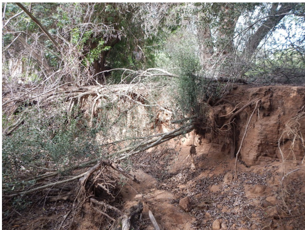
Fig. 7 Typical southern California example of incision and bank failure observed in fine-grained channels downstream of conventional development (27% TIA, developed in the 1980's) that lack stormwater intervention tailored at reducing sediment transport capacity
