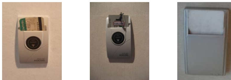
Wrong replacement by parking ticket and other cards
