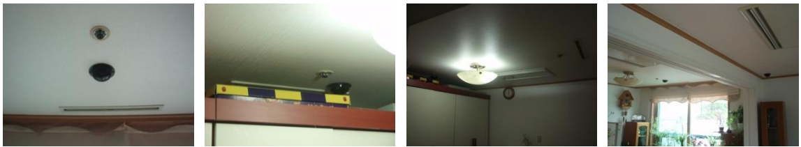
CCTV in bedrooms and living rooms
