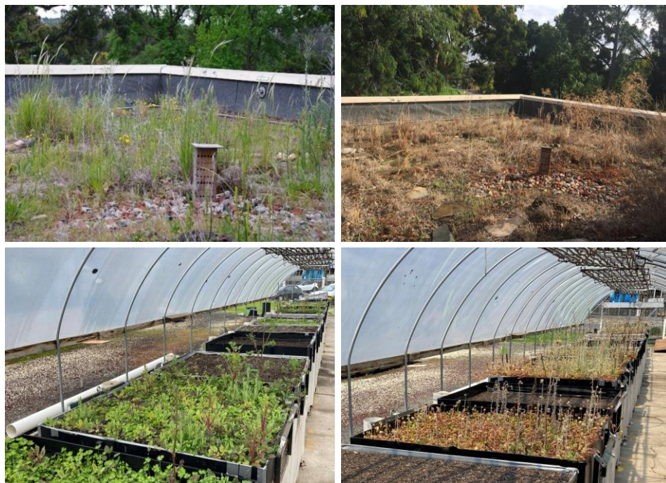
Figure 7.2 Green roof vegetation exhibits dynamic changes regardless of initial design, especially under varying water availability. Clockwise from top left: Burnley biodiversity green roof in Spring 2016; the same in Summer 2020; green roof modules in the 'dry' regime from Chapter 5's stormwater experiment; and the same modules in the 'wet' regime.
