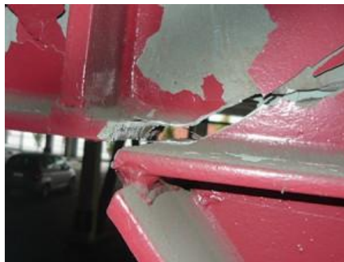
Figure 2-63 Brittle failure at a connection [76]
