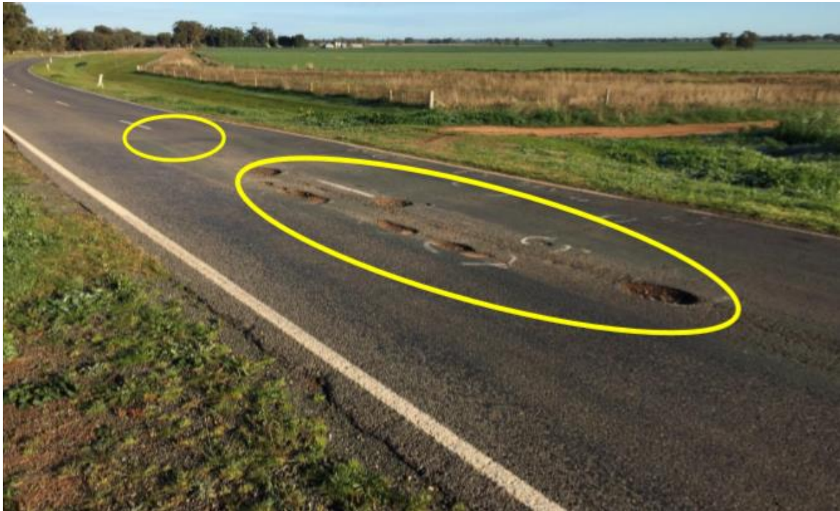
Figure 3.4: Subsurface damage of a road
