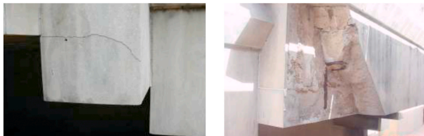
(a) Cracking of limestone unit and spalling area (b) Corroding of fixing cramp
