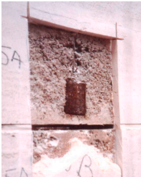
Fig. 2. Embedded corrosion of steel anchor plate in precast concrete wall [2].
