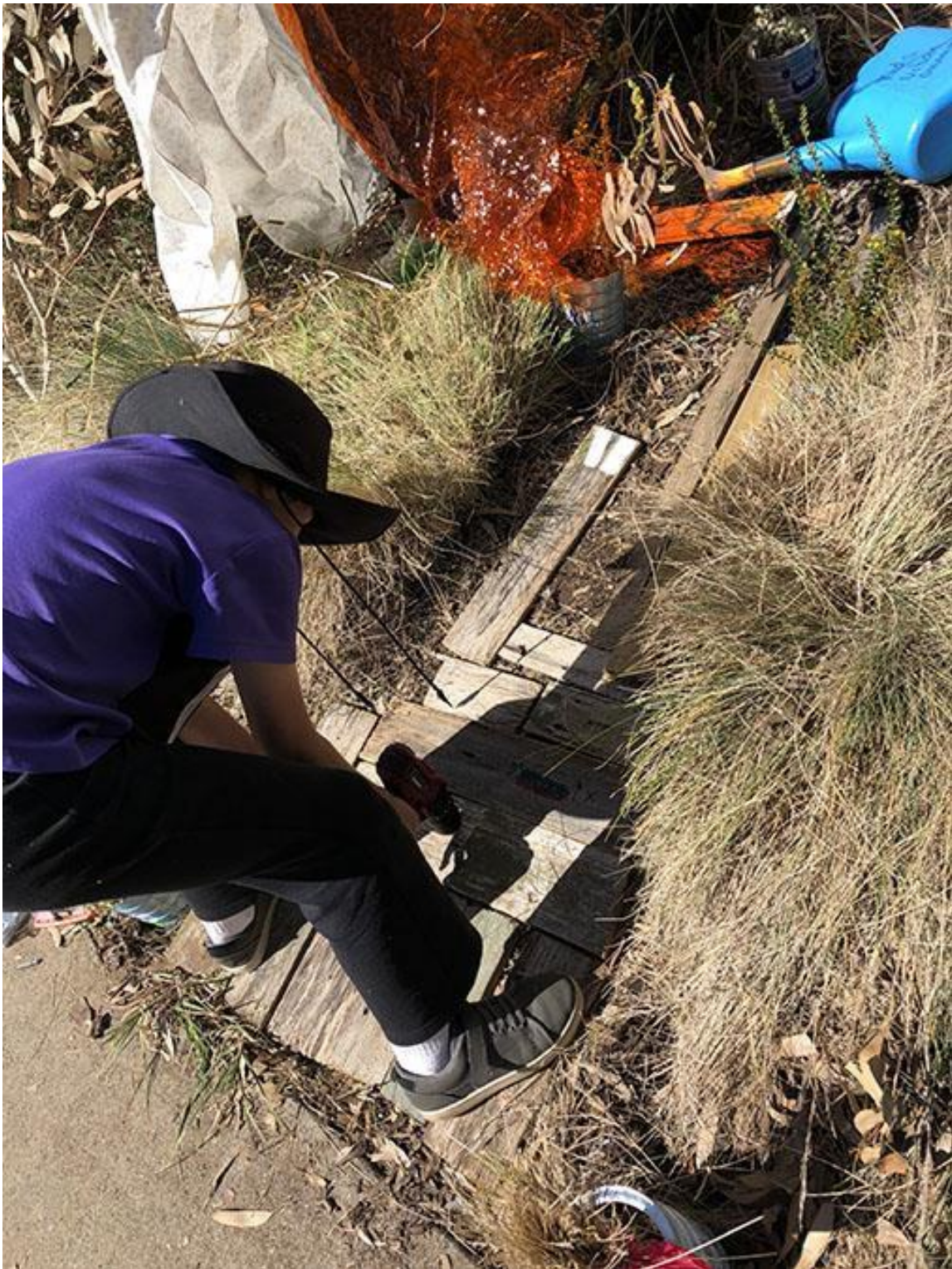
Figure 33: Steps being reconfigured to create a pathway at Campus 2 Image by: Clare Walton 2018
