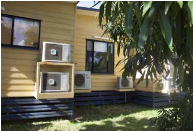
FIGURE 7 Air-conditioning units mounted onto prefabricated housing designed and prefabricated by Ark manufacturers in Queensland in Nhulunbuy. Source: Author, 2015.
