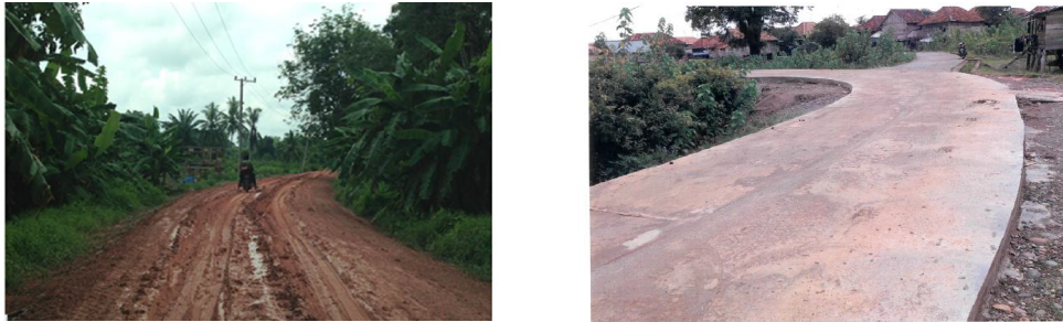
Figure 6.4. Road conditions before and after community protests
