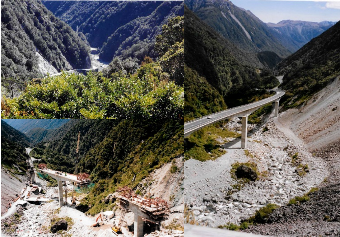
Figure 1: Construction of the Otira Viaduct, NZ: Before (a), during (b), and after (c). Source: West Coast New Zealand History (8th Oct 2016). Photo's [sic] of the old road Otira Gorge and the building of the viaduct. Photographer: Don Hutton. In Website West Coast New Zealand History. Retrieved 9th Oct 2019 15:29, from https://westcoast.recollect.co.nz/nodes/view/12762
