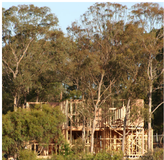
Development in urban fringe areas highlights the vital role urban planning can play in improving the survival of dwellings in bushfire events.
