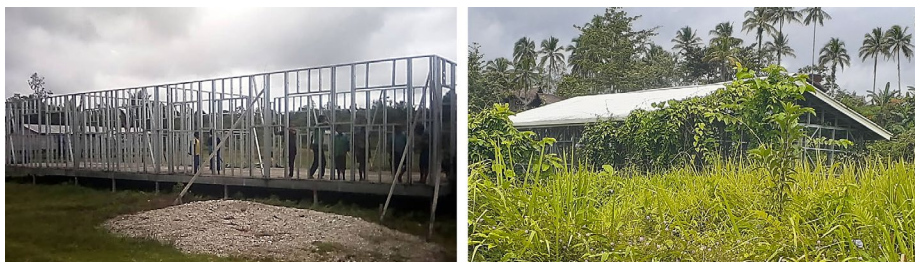
FIGURE 1 Two failed projects at Soabi in 2023—the 'naked building' (planned duplex classroom) and the 'kunai haus' (planned new aidpost building).
