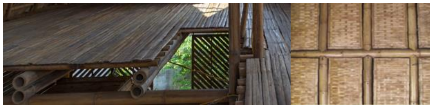
Figure 5: Example of flooring and a wall structure using cut bamboo poles (Sources: H&P Architects and Minke, 2012).
