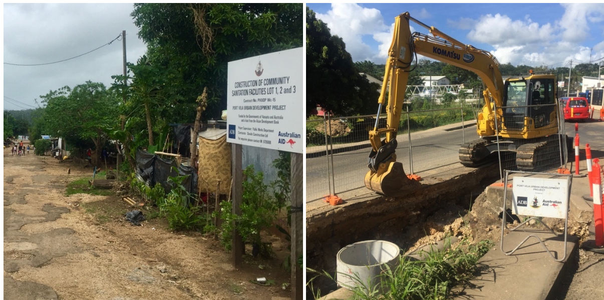
FIGURE 5.9: COMMUNITY SANITATION FACILITY DEVELOPMENT WORK IN SEASIDE (LEFT) & TRUNK DRAINAGE INFRASTRUCTURE UPGRADING (RIGHT) IN CENTRAL WARD
