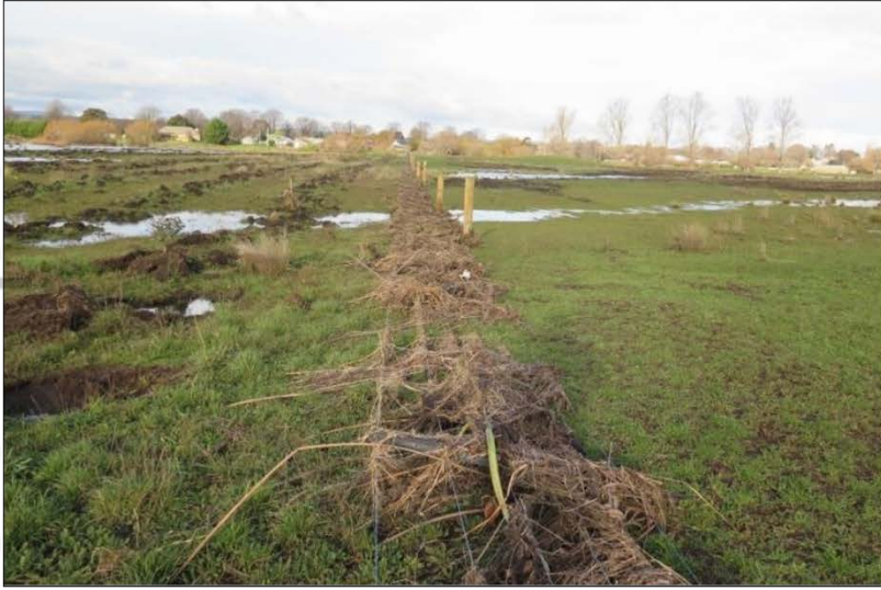
Figure 3. Flood damage to a riparian fence, Macquarie River, Tasmania (Photo courtesy of Jimmy Collinson, Greening Australia). This fence would most likely need to be replaced.
