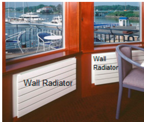
Figure 2. Good view factor between wall radiators and body of occupant seated on chair.
